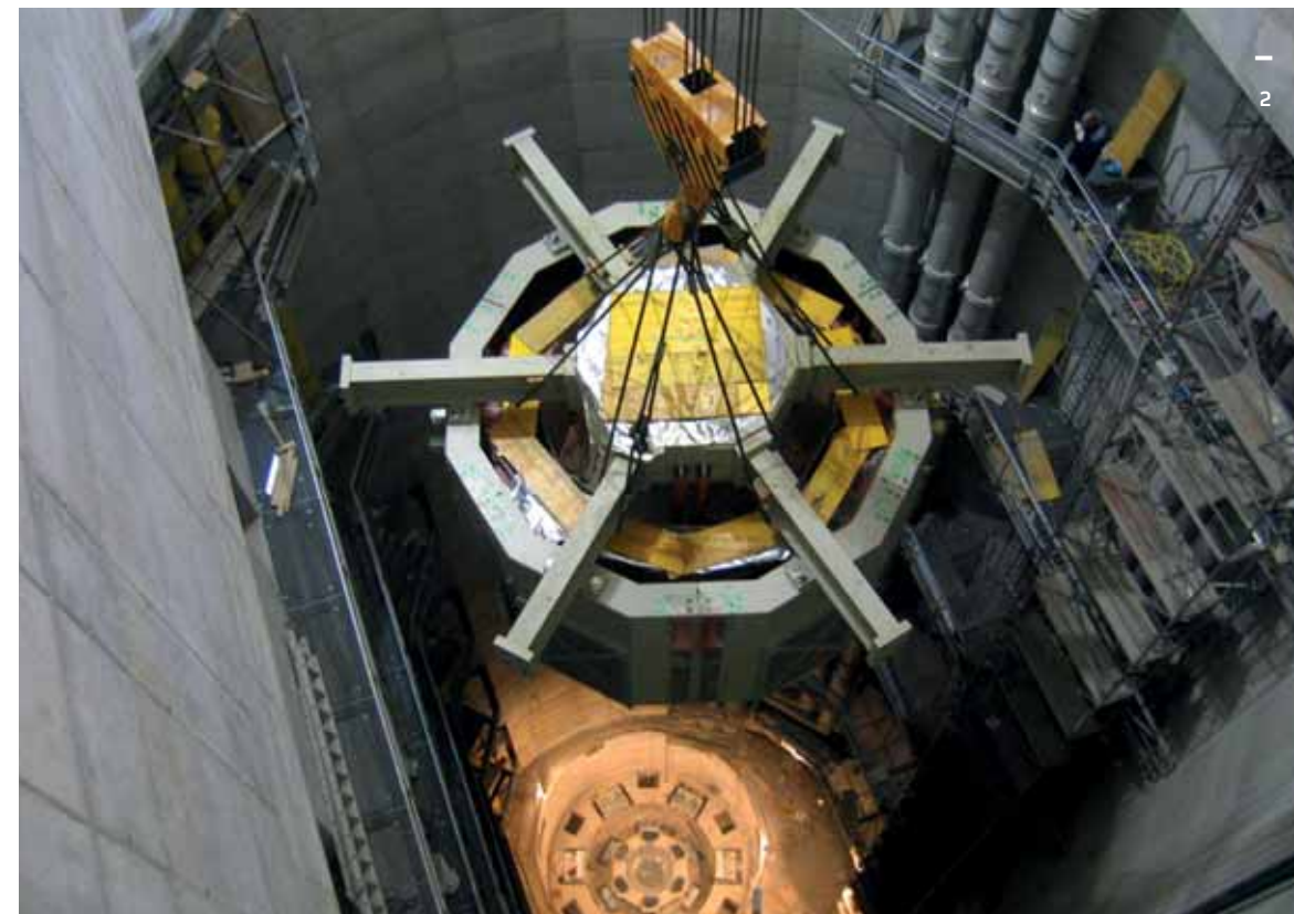
2_ Spust statorja v strojnični jašek 2_ The launching of the stator into the powerhouse shaft
